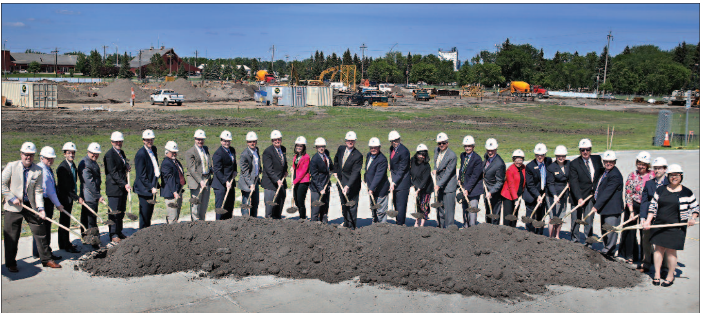
The University of North Dakota held a ceremonial groundbreaking for the new $122 million School of Medicine and Health Sciences building on June 12. Governor Jack Dalrymple, Senators Ray Holmberg, Robert Erbele, Judy Lee, Grand Forks Mayor Michael Brown, Altru Health System CEO Dave Molmen, UND President Robert Kelley, and SMHS Dean Joshua Wynne provided remarks on the effect the new building will have on healthcare training in the state.
