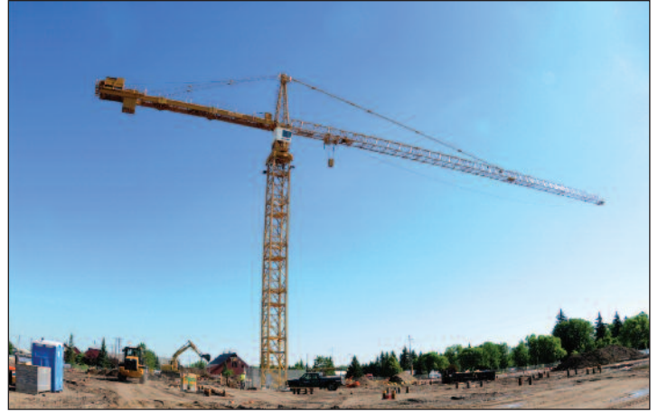
On June 20, the tower crane that contractors will rely on in the construction of the new SMHS building was up and running.
